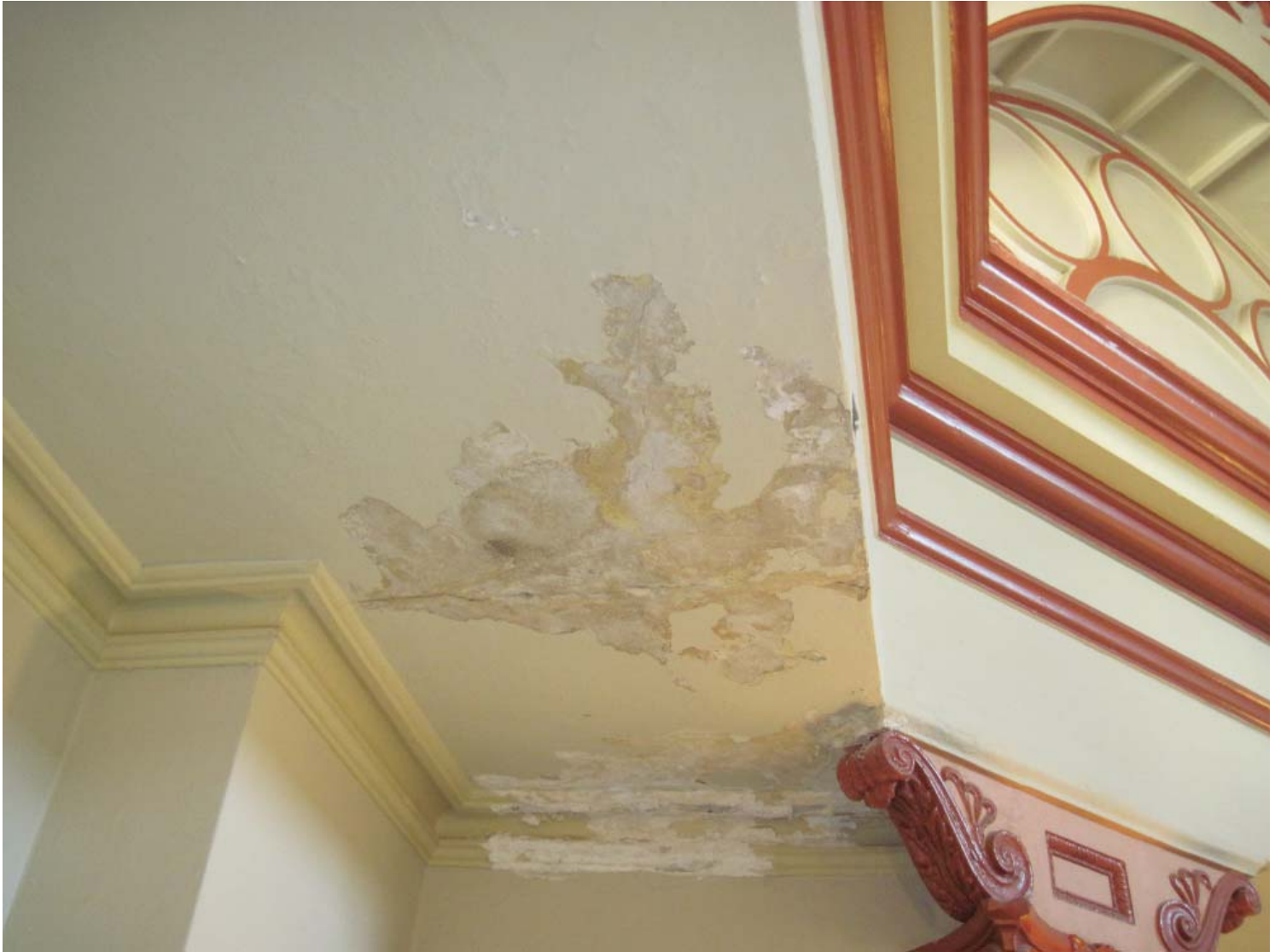
1) Leakage from outside along window in rotunda has caused plaster damage in picture above.
