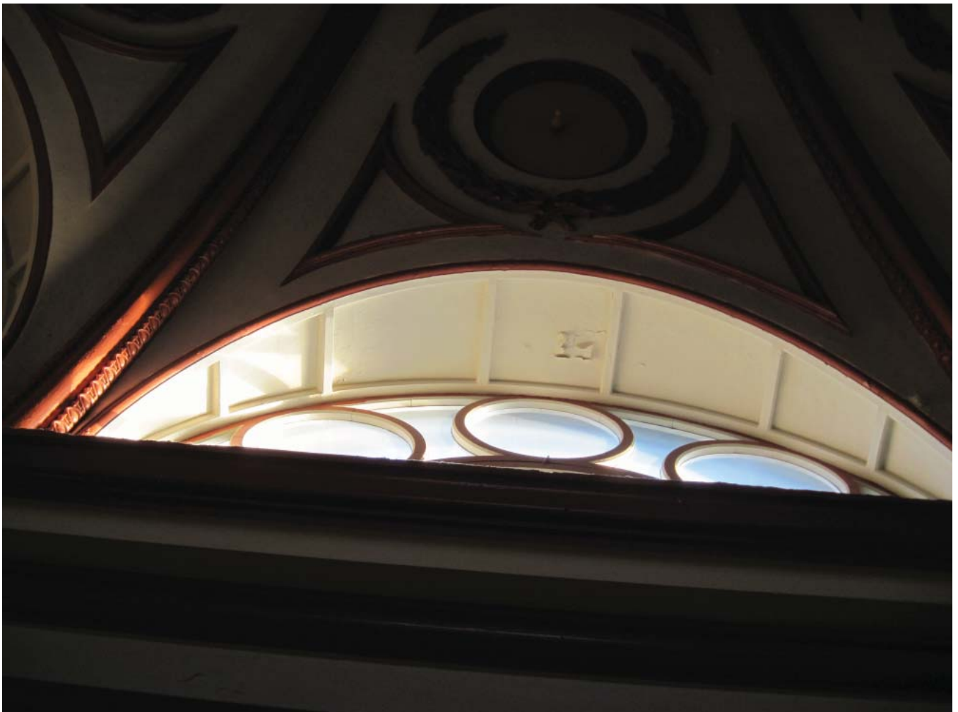
2) Leakage from outside along window in rotunda has caused plaster damage in picture above.
