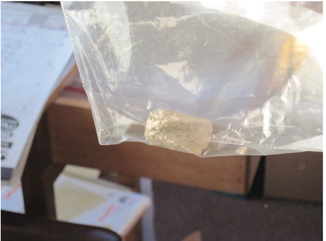
Pic #10. Masonite ceiling tile piece that has fallen from the ceiling
